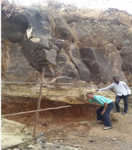
Figure 4: Weathered materials of basalt at bottom (mud basalt) getting removed or washed out leaving its space to be filled by overlying basalt causing landslide or submergence
