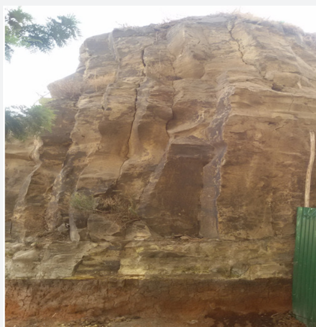
Figure 2 :Weathering of basalt at the bottom under continued wetness caused by accumulated rainwater through the vertical space or cracks in basalt rock.
