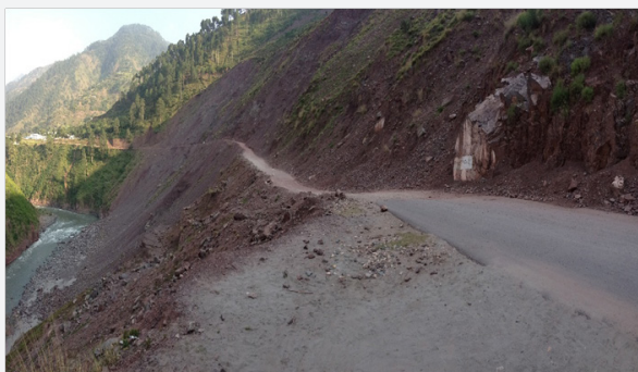
Figure 5: Devlian landslide on Neelum Valley Road.
