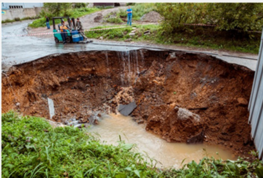
Figure 17: A hole several meters deep has formed on Shoshina Street in Vladivostok.
