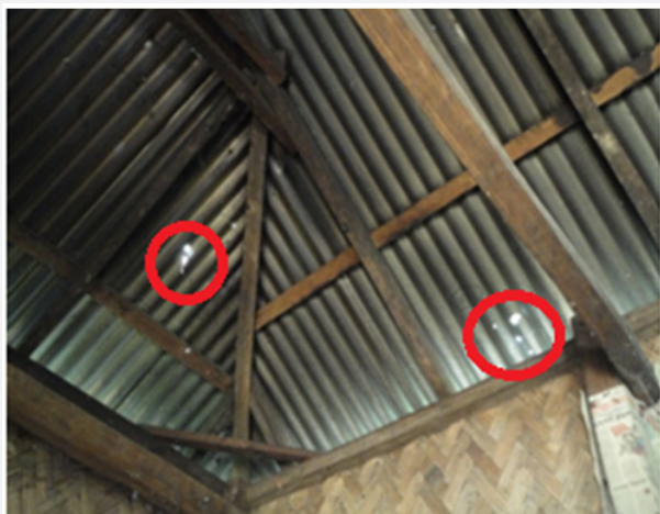
Figure 7: Overted five holes caused by bullet/fragment on tin roof.
