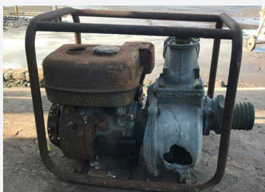
Figure 5: View of centrifugal pump with an irregular hole.
